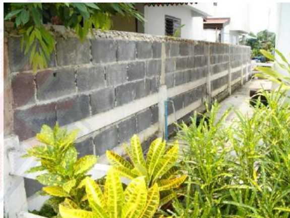
Figure 7-3: The original fences (the lower white lines) were widely changed in the NHA Rangsit Klong 3 community
